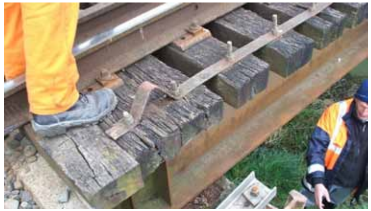
Damage to Bridge 18 on the Main North Line, shows the force of the quake on rail structures.
