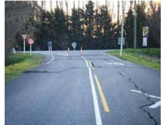
Damage to the road at the approach to a level crossing.
