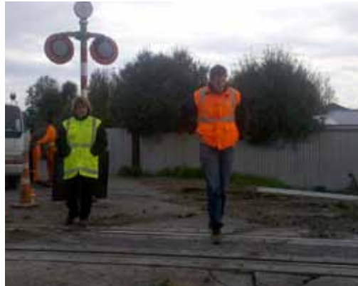
Bronwyn Woodham and Todd Moyle inspect the damage at a level crossing in Kaiapoi.
