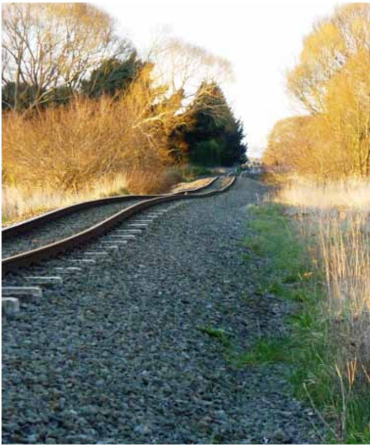
Above: Dropped tracks south of Bridge 18 which use to be straight and level. Below: The 'ramp' up to the bridge again showing just how much tracks dropped in the earthquake.
