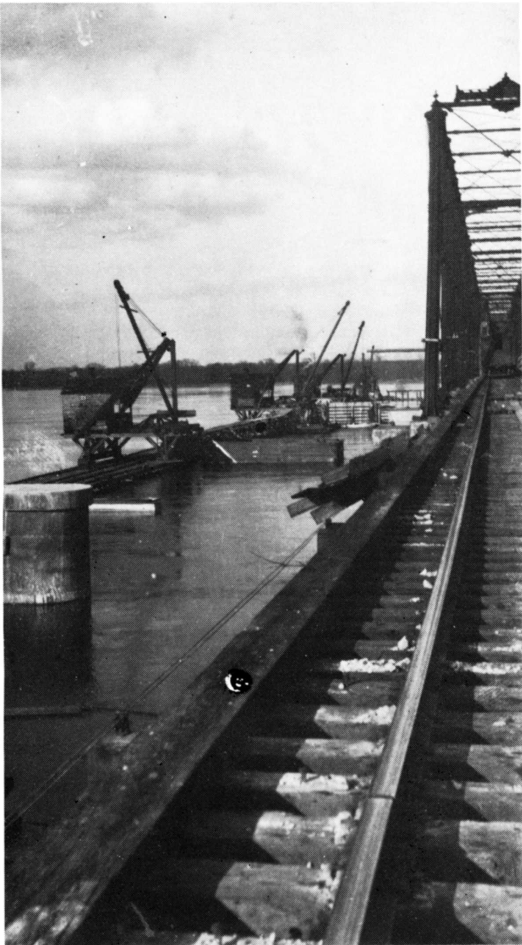
While the ornate old bridge continues in service, steam cranes prepare coffer dams in preparation for pouring concrete abutments for the new bridge. Collection of Gus Hart.
